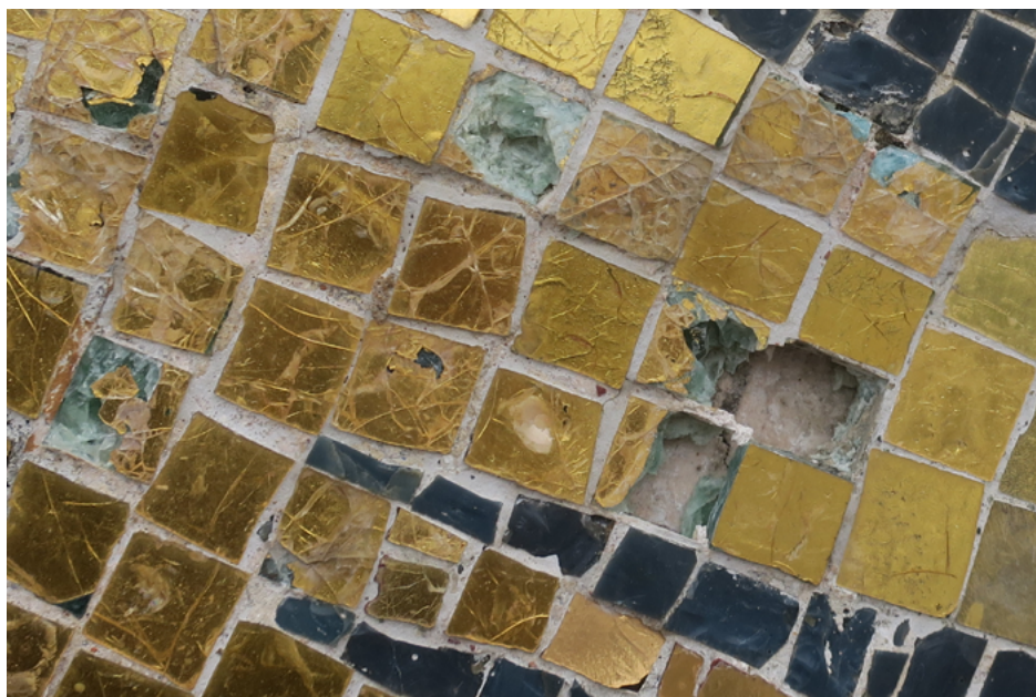
Damaged gold smalti after a hailstorm (photo Malu Storch)
