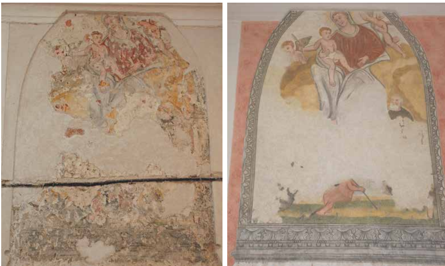
Fig. 1c: The Madonna and Child on the northern presbytery wall of St Nicholas's Church in Kred before and after the presentation. The retouch extends into the loss and so optically lessens it. The preserved wall painting is in the foreground. The decorative frame of the scene is reconstructed.
