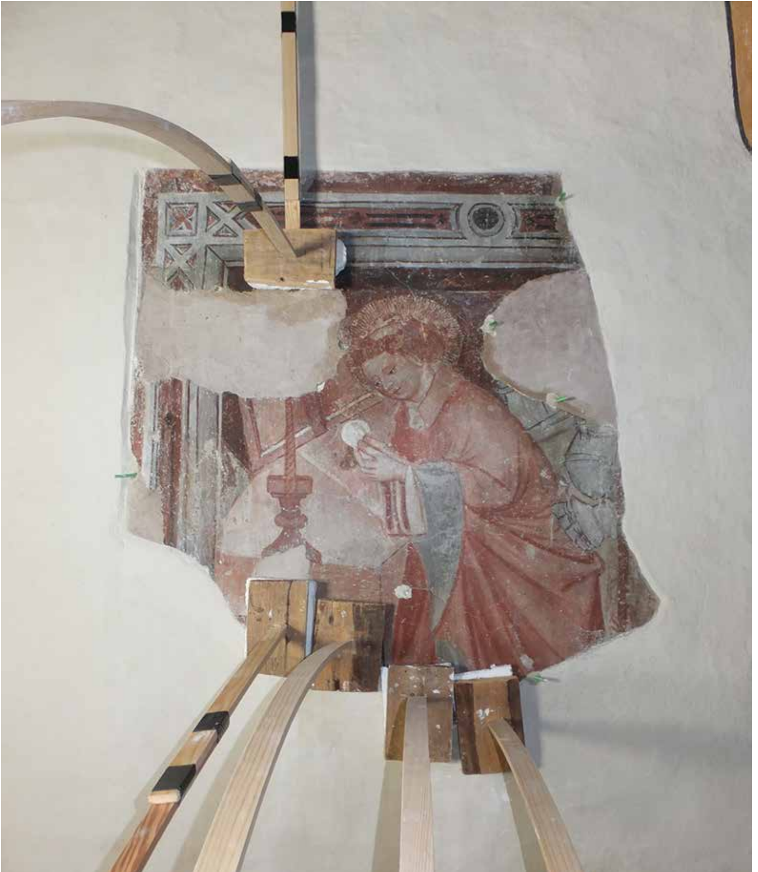
Fig. 10: Protective works on the southern presbytery walls of the parish church in Hermagor (Šmohor) in the scope of the July 2018 monitoring.
