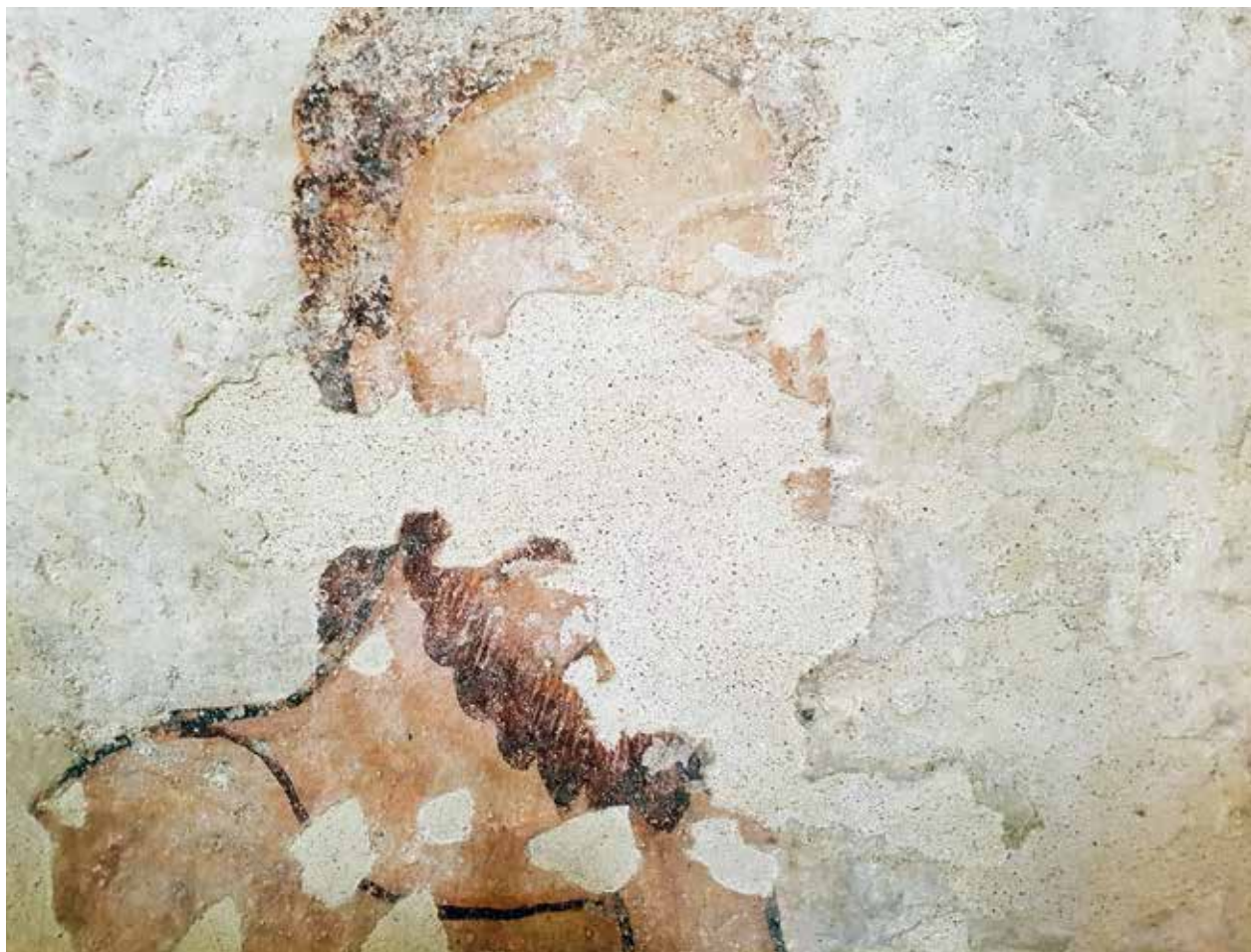
Fig. 9: In St Jacob's Church in Urschalling the gap that could not be reconstructed was filled with toned plaster below the painting level.
