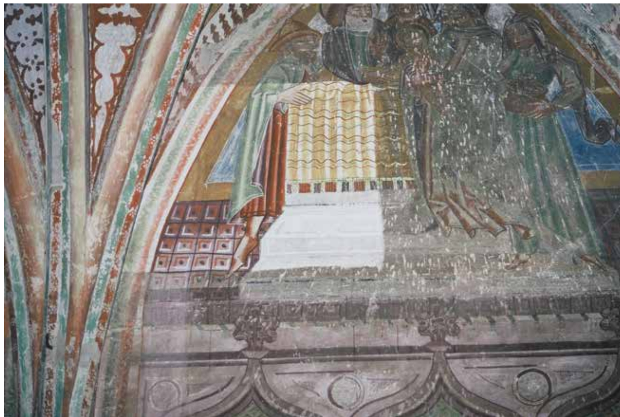
Fig. 1: An example of severe dirt and mould on the wall painting by the master of Suha from the mid-15th century in the St John the Baptist parish church in Suha near Škofja Loka. The test dirt removal probe shows the colourfulness of the original.
