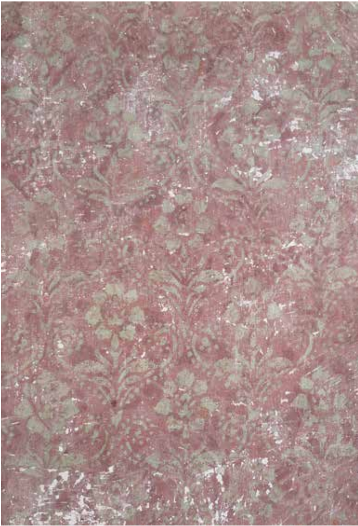
Fig. 1: After probing and initial uncovering of the paintings in the Tavčar Manor in Visoko near Poljane, we assumed that the green pattern was painted on a dark red background, which is an interesting but rather strange hue combination.
