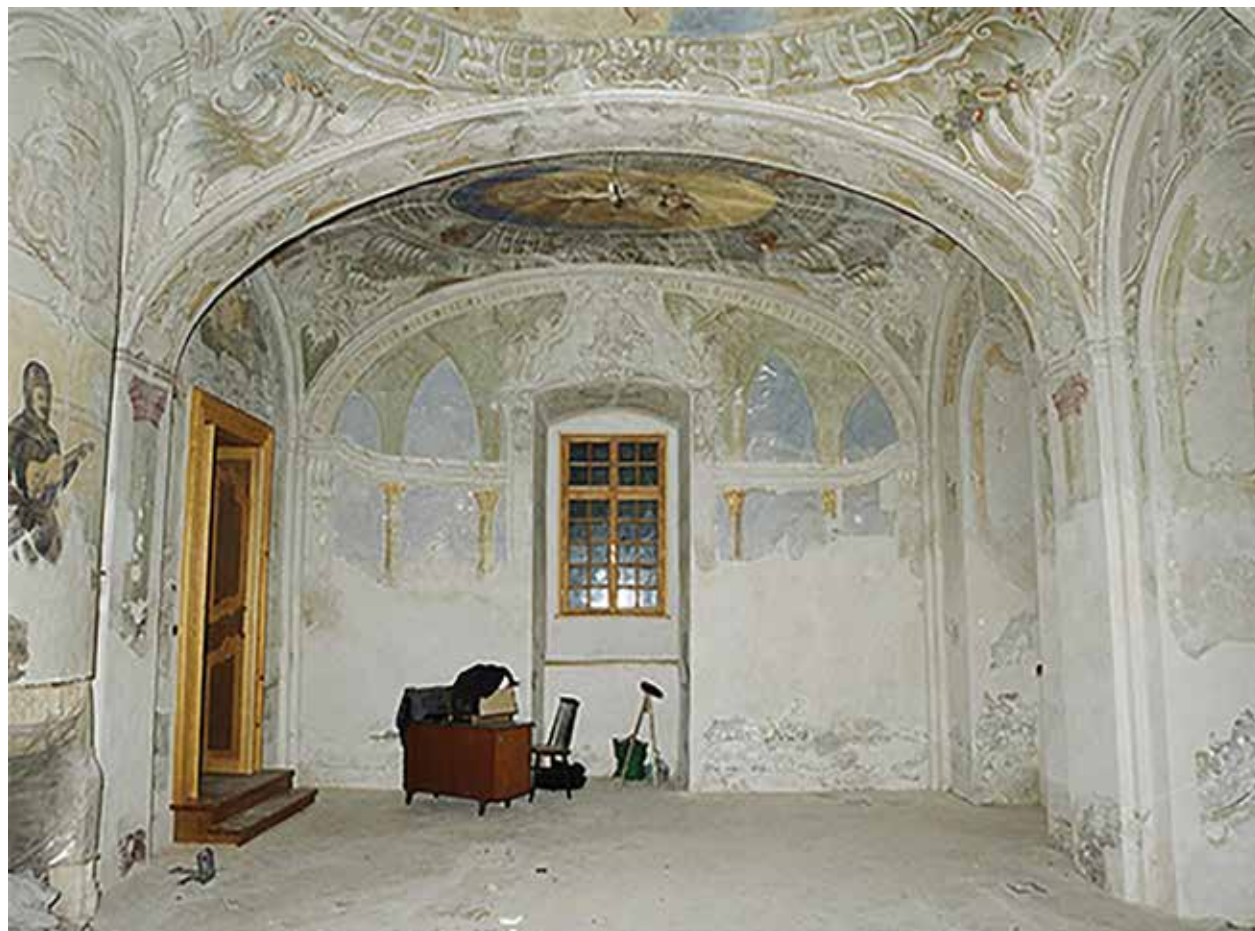
Fig. 5: Salle terrain before the restoration treatments in the south auxiliary house of the castle Batthyány in Ludbreg (painted c. 1762).
