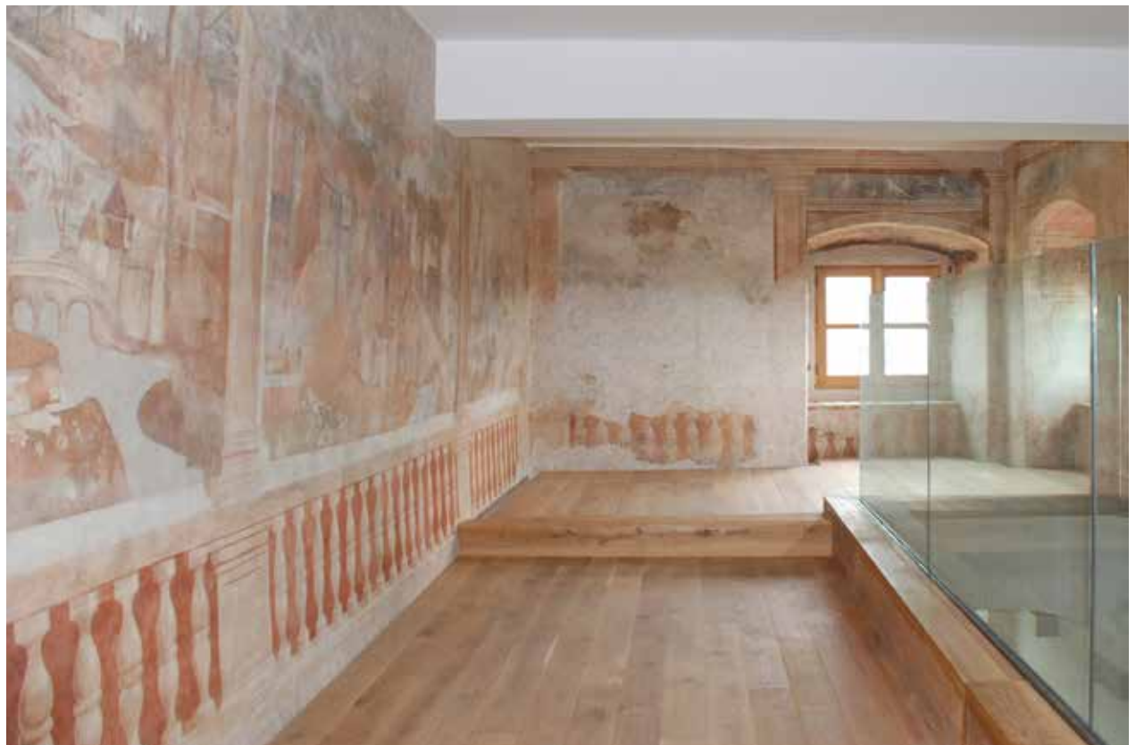
Fig. 4a, 4b: The painted space in the Vipolže Villa before and after the intervention. The losses in the plaster were puttied in level with the painting and toned with light-toned paints applied with sponges resembling the surrounding painting to make them less noticeable and disturbing.
