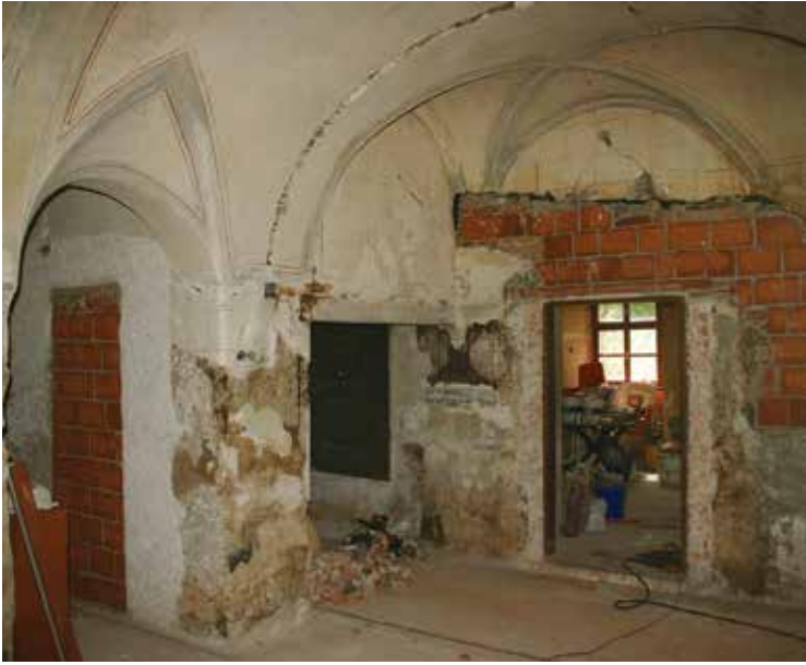
Fig. 3: The state of the painted room in the Tavčar Manor after the removal of the secondary layers and the weathered and inappropriate plasters.
