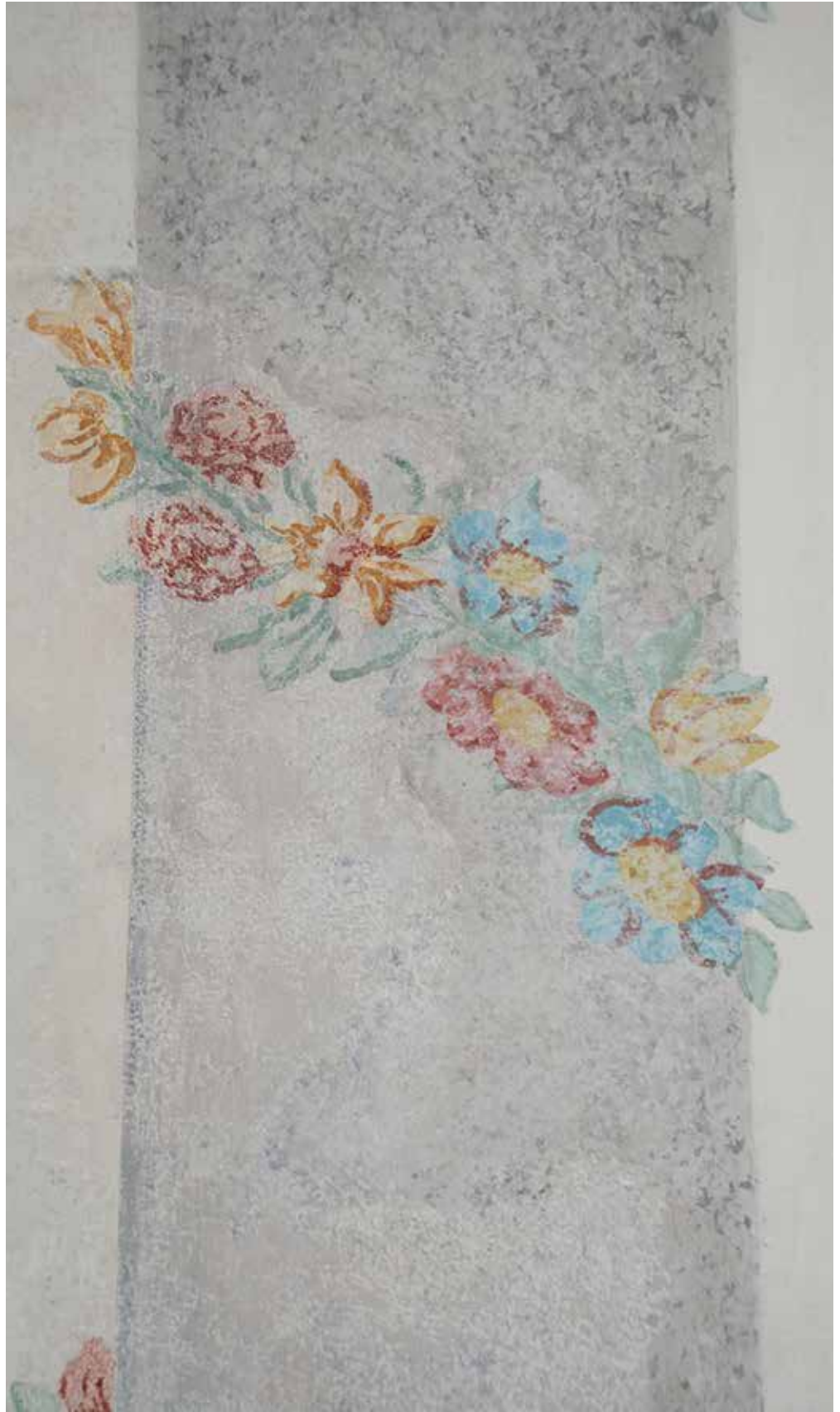
Fig. 6: The lower left section of the painted column from the Lanthieri Manor in Vipava is the original retouched with dots. The upper right section is a reconstruction in limewash. The plaited plants and flowers were reconstructed with matrices and later shaded by observing the original.
