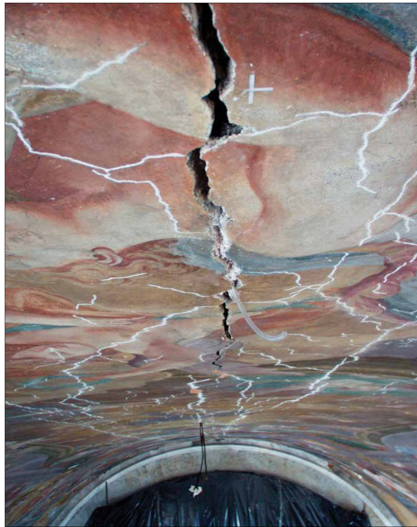
Figure 74: Wide longitudinal cracks on the apex of the vault.
