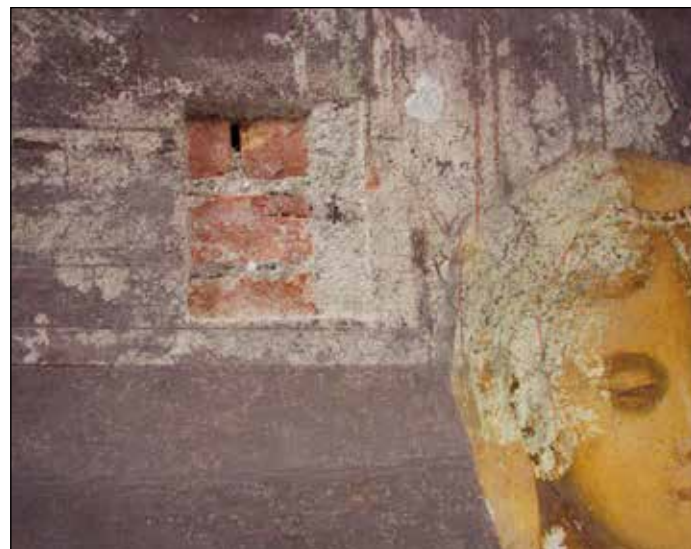
Figure 23: Damaged surface of the vault painting (location H19).
