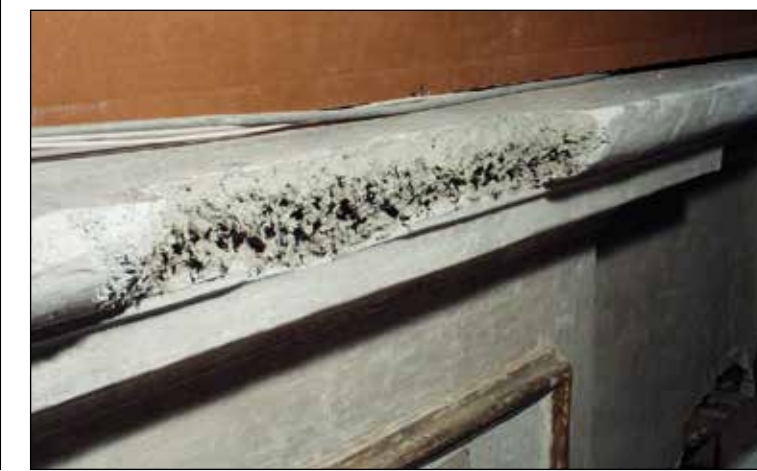
Figure 29: The application of a new binding mortar at the beginning of the reconstruction of the cornice.
