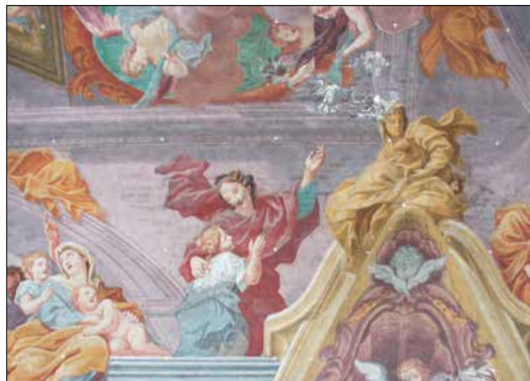
Figure 235: Condition before treatment – a large area with visible signs of leakage.
