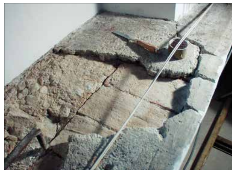
Figure 27: The window sill beneath the vault window where the brick construction of the profiles is visible.
