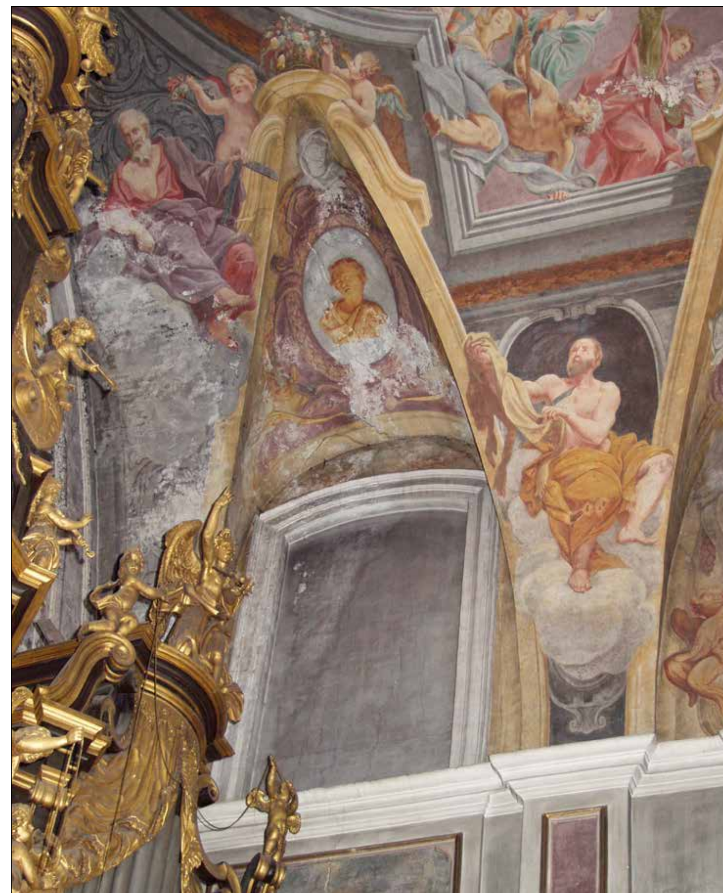
Figure 92: North-western corner – results of leakage.
