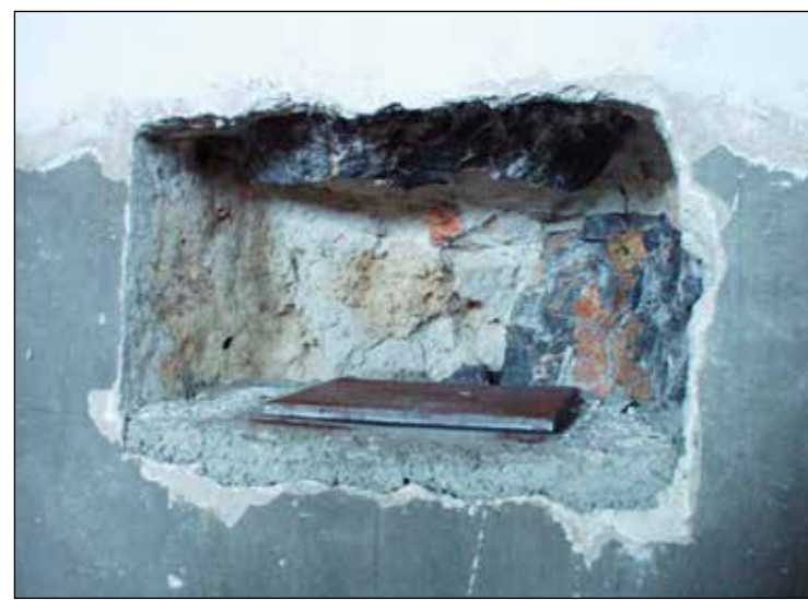
Figure 28: Damage occurred with the anchoring of the restoration platform.
