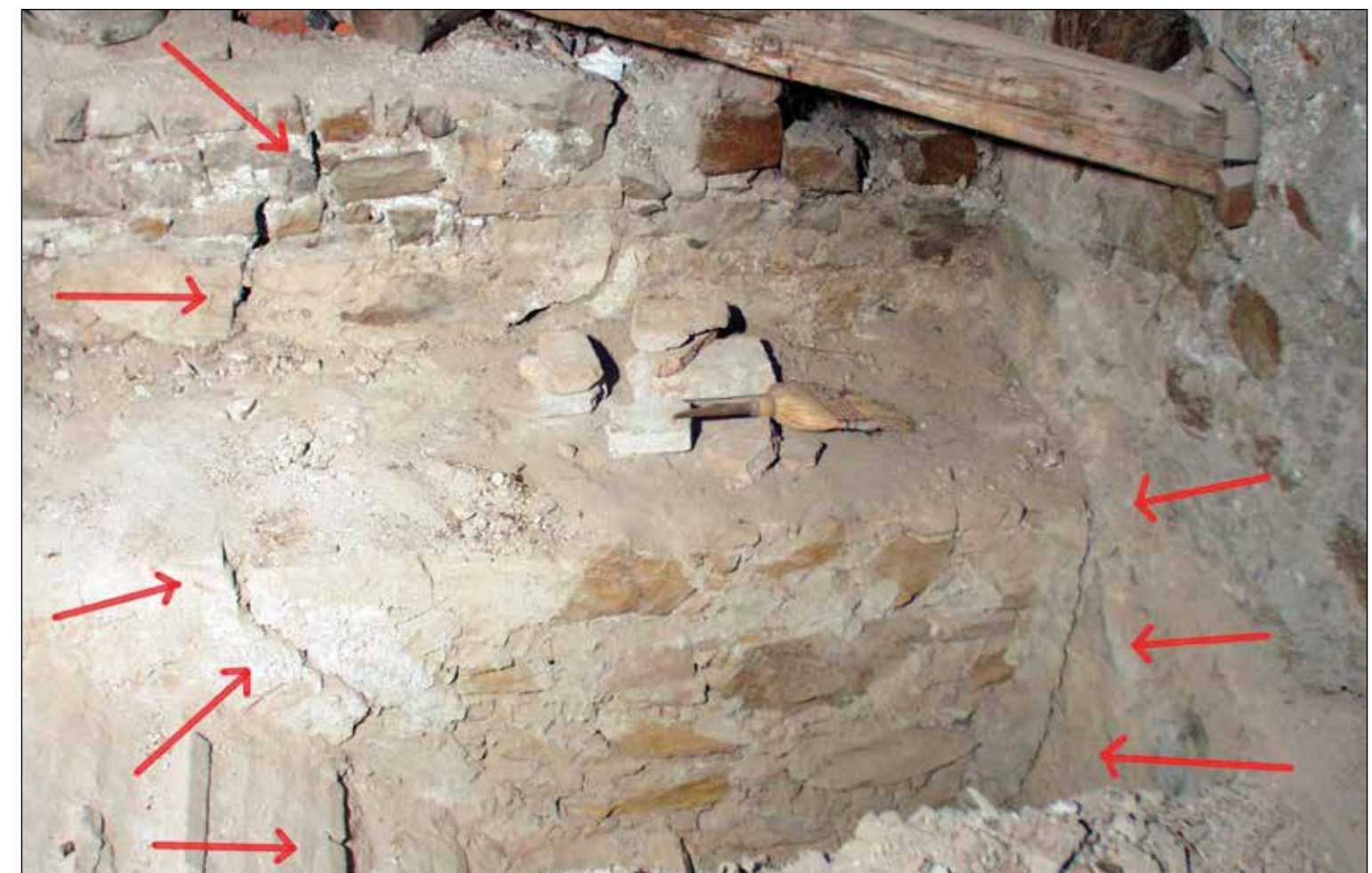
Figure 38: Testing probe in the north-western corner of the attic with marked arrows indicating a large crack on the left and detachment of the masonry.
