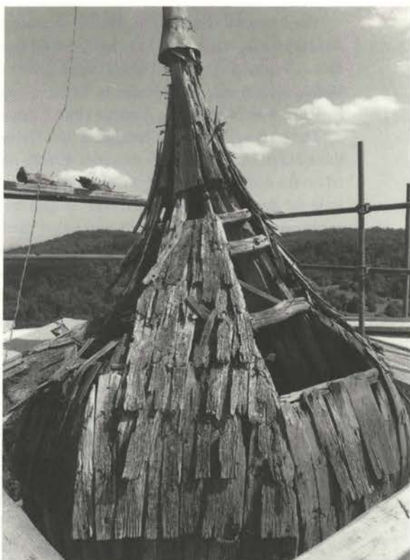
Dilapidated roof of the bell-tower: "The utterly decayed roof construction and covering of the Baroque cap of the bell-tower were replaced in that year (i.e. 1987)."
