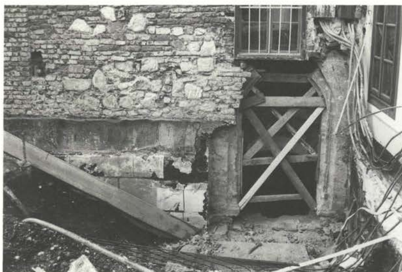
Gothic portal before the renovation: "The discovery of the external Gothic portal posed a somewhat greater dilemma, since it was located 1.5 m below the level of the square, therefore requiring intervention in the present regulation of the urban setting."
