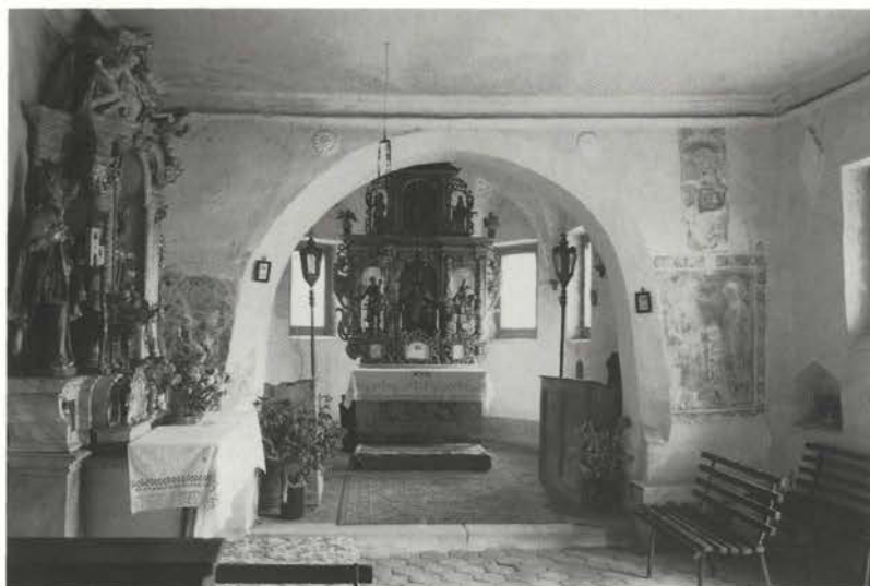
Interior of the church: "After renovation of the plasterwork on the facades and in the narthex, the work was continued in the interior of the church..."
