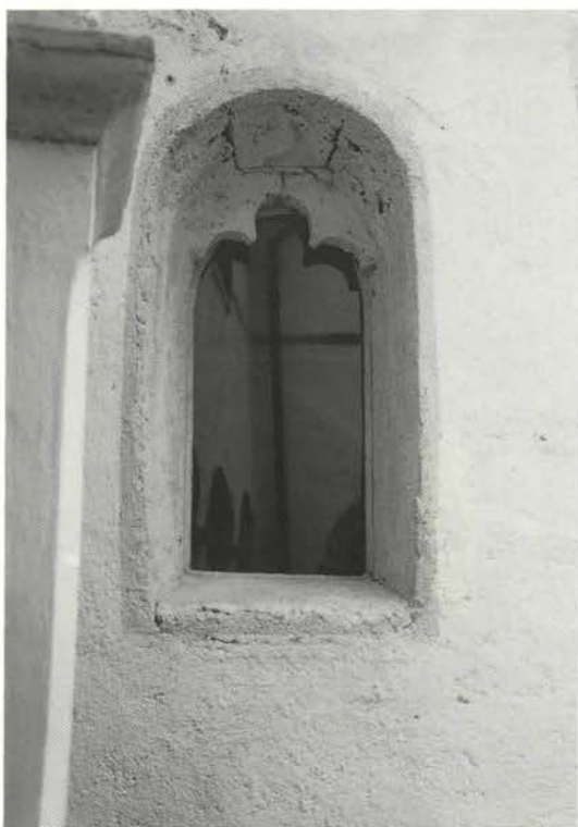
Renovated Gothic window: "The removal of the staircase facilitated the discovery of a small Gothic window with a trefoil conclusion on the western facade of the turret."
