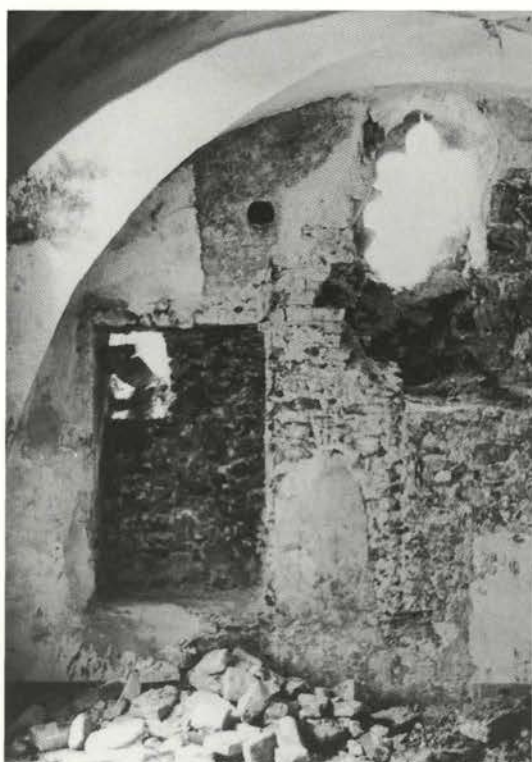
View from the inside: "The north-eastern turret – the opening up of a Gothic window with a trefoil conclusion..." .....
