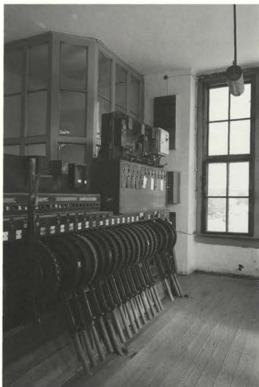
Interior of the signal box: "A complicated system of wheels, guides, conduits and brackets connected the switches mechanically with the control lever mechanism in the tower." .....
