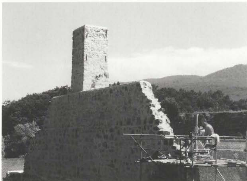
Renovation of the north wall. "In 1994 the second phase of the renovation of the former ironworks took place..."
