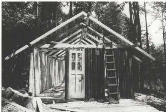
Hut No. 19 during the renovation. "In January 1995 a tree uprooted by strong wind leaned on the hut..."
