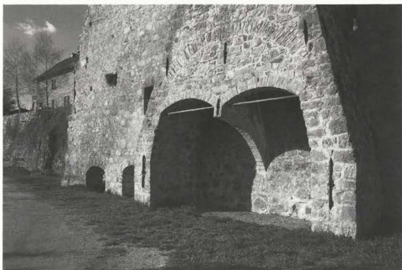
Renovated remnants of the chimney stack of the furnace. "The decision was taken to renovate two brick arches with primarily structural functions on the lower part of the wall..."
