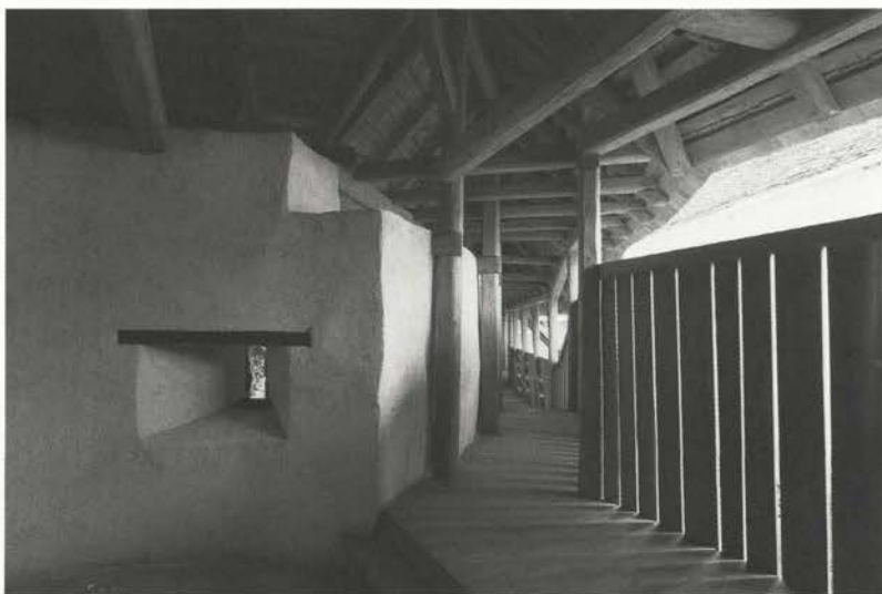
View along the wooden defence parapet. "The starting-point for the preservation and reconstruction of the entire walls was the well-preserved embrasures on different levels..."
