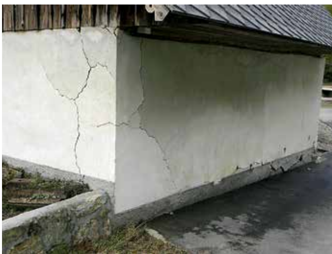
Hotovlja, Fortunov mlin in kozolec, poškodovana stena mlina (foto: D. Pediček, 2014)
