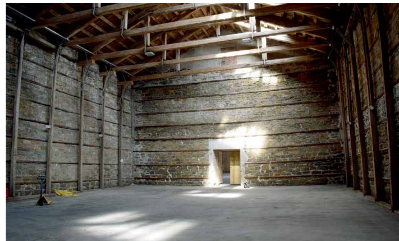
5. Notranjost 2. kampaite skladišča Monfort, brez stenskih oblog (foto: Ana Plestenjak) 5. Interior of bay 2 of the Monfort warehouse, without wall cladding. Photo: Ana Plestenjak
