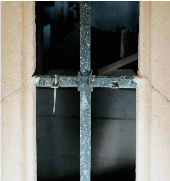
3. Muta, cerkev sv. Janeza Krstnika, detajl originalnih kovanih prečk v južnem oknu (foto: Robert Peskar) 3. Muta, St. John the Baptist's Church, detail of original wrought glazing bars in the southern window (Photo: Robert Peskar)
