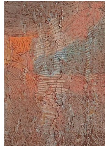
4. Anton Cebej, Križev pot, XIV. postaja. Razpoke na kitu (foto: Anka Batič) 4. Anton Cebej, Stations of the Cross, 14 th Station. Cracks in the filler (photo: Anka Batič)
