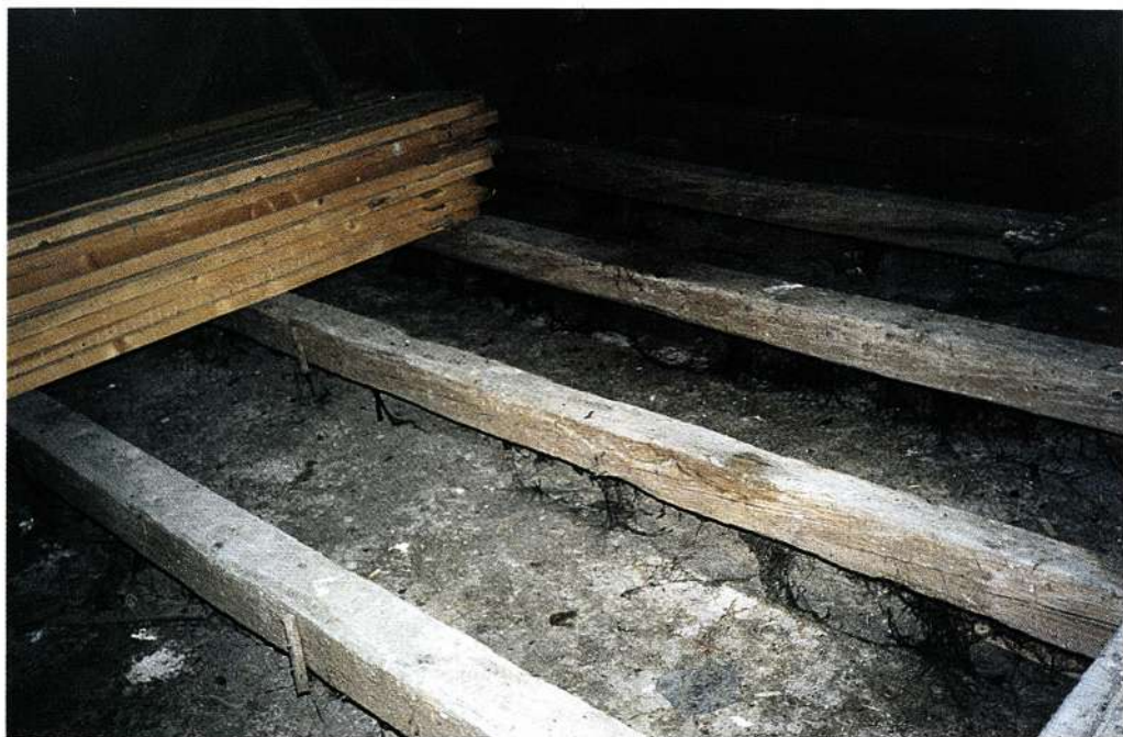
Podstrešje z ostanki čepasto prirezanih poveznikov, ki so nekdanj nosili leseni strop. Vse fotografije Uroš Lubej. Attic with remnants of wooden joints cut like bungs, by means of which the wooden ceiling used to be hung. All photographs by Uroš Lubej.
