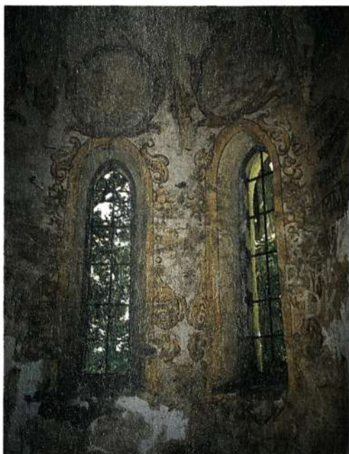
Poslikava v prezbiteriju pred restavriranjem Decorations in the presbytery prior to restoration
