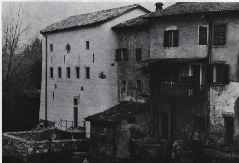
Sl. 64. Kanal, Pionirska 8 – stanje po obnovi – vzhodna fasada in zahodna fasada Fig. 64 – Kanal, Pionirska 8 – situation after renewal – eastern façade and western façade
