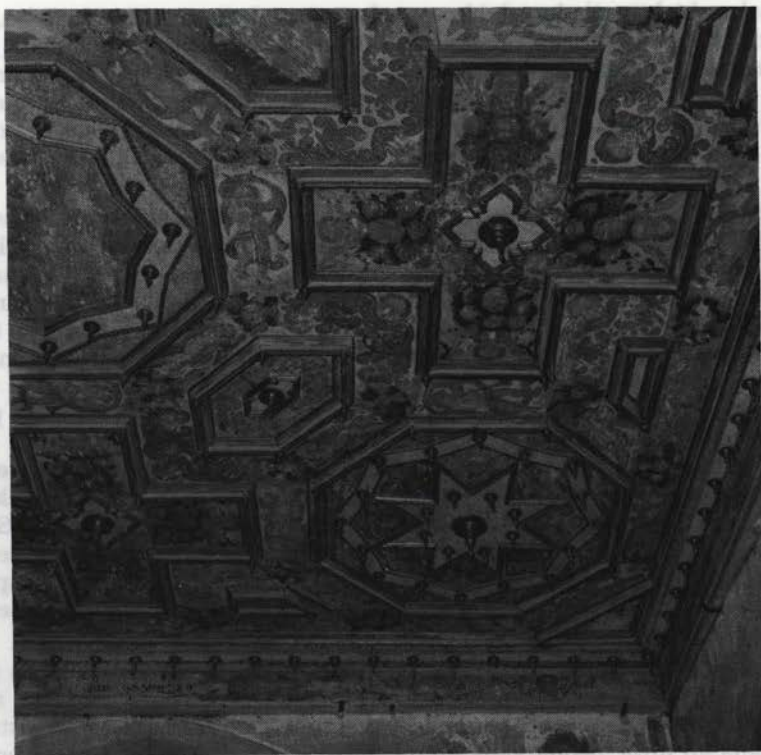
Sl. 72. Gostče, leseni strop po obnovi (f. V. Benedik) Fig. 72 – Gostče, the wooden ceiling after restoration
