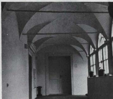
Sl. 114 b, c Celje – Tomšičev trg 1, hodnik med in po obnovi Fig. 114 b, c Celje – historic centre, the corridor in one of the houses
