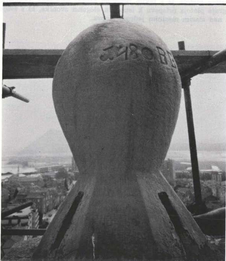
Sl. 56. Koper, kamnito jabolko na vrhu stolpa. 1480 je letnica najstarejše znane obnove Fig. 56 — Koper, the stone apple at the top of the belfry. 1480 is the date of the oldest known restoration
