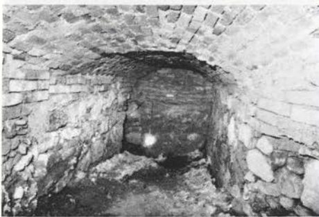
Sl. 34. Celje — kanal z opečnim obodom, zadaj, levo starejši, kamnit kanal Fig. 34 — Celje — sewer with brick circumference, at back, to the left older, stone-made sewer
