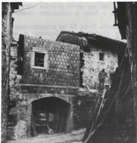
Sl. 2. Goče — stavbni niz med obnovo Fig. 2 — Goče — a string of buildings during restoration
