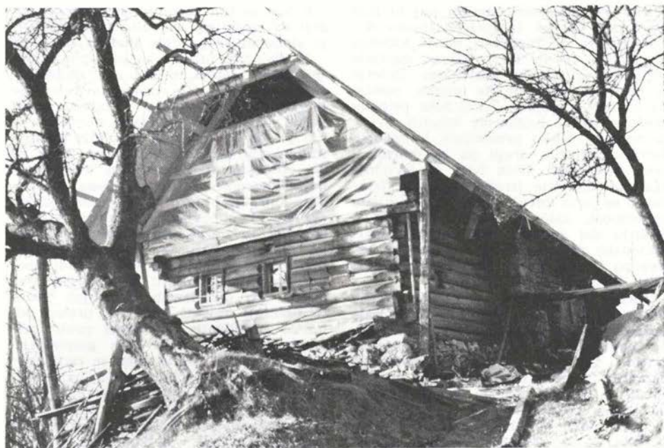
Sl. 26. Zg. Palovče — pogled na Budnarjevo hišo med deli Fig. 26 — Zg. Palovče — view of the Budnar house during the works
