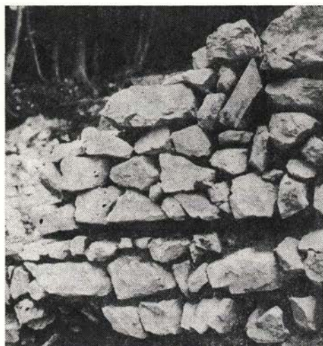
Sl. 22. Ajdna — nivo prvotnega cerkvenega praga, viden v strukturi zahodnega zidu Fig. 22 — Ajdna — level of the original church threshold, visible in the structure of the western wall
