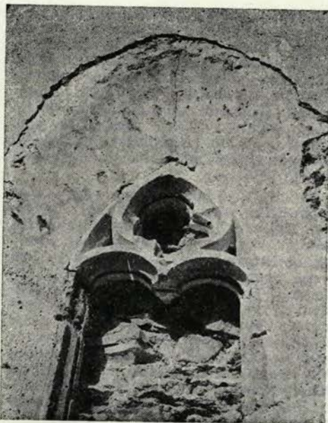
Sl. 107 Arnače, ž. c. sv. Ina — novo odkrito gotsko okno v vzhodni steni prezbiterja Fig. 107 Arnače, the parish church of St. Egidius — the newly discovered Gothic window on the eastern wall of the presbytery
