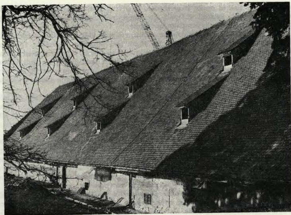
Sl. 39 Ptuj — na novo prekriti južni del strehe na bivši grajski žitnici Fig. 39 Ptuj — the newly covered southern part of the roof on the one-time castle granary
