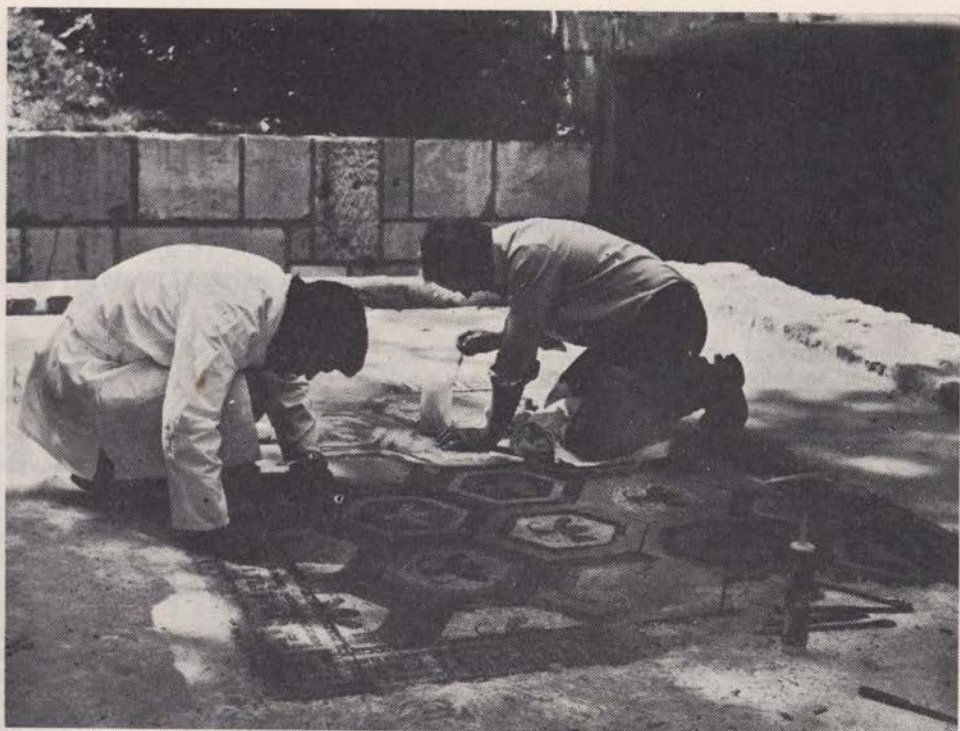
Sl. 11 Pogled na mozaično površino med fugiranjem. Okrog mozaika je že imitacija estriha Fig. 11 A look at the mosaic surface during jointing, around the mosaic being already the imitation flooring
