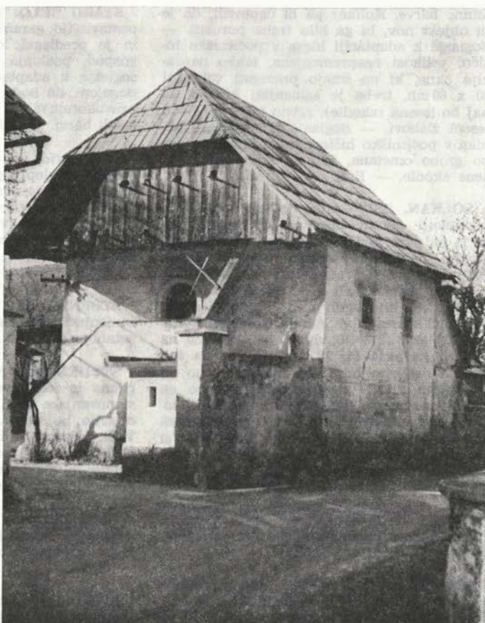
Sl. 35 Pristava pri Tržiču, baročna kašča s poškodbami zaradi prometa Fig. 35 Pristava near Tržič, The Baroque granary, damaged on account of the traffic
