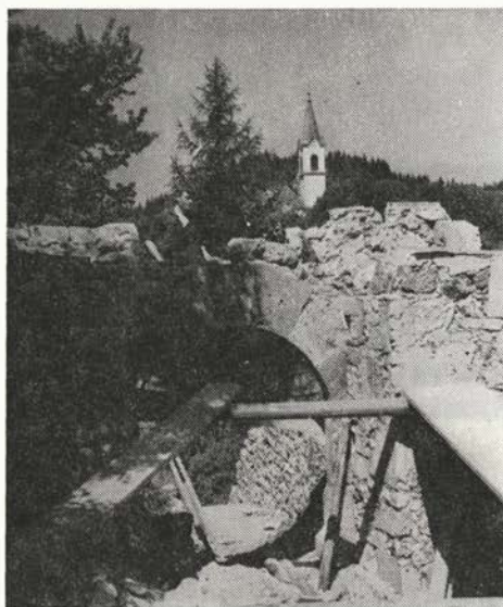
Sl. 21 Kamnik, obnavljanje Veronikinega portala na Malem gradu Fig. 21 Kamnik, Reconstruction work of Veronica's Portal on the Small Castle Hill
